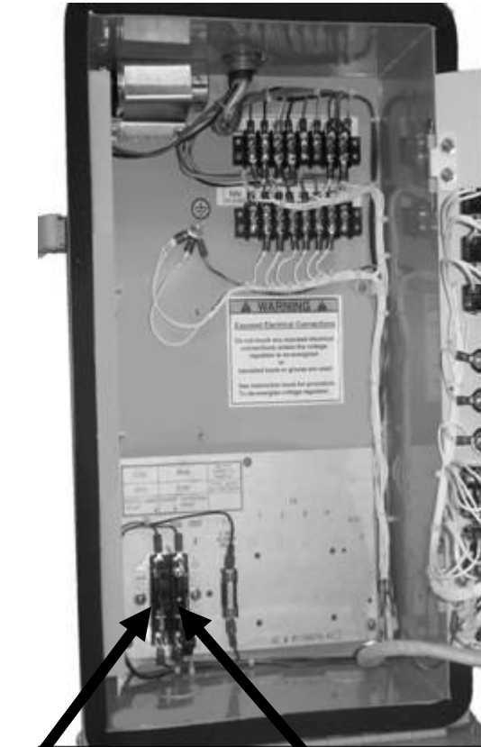
PT Disconnect Switch
