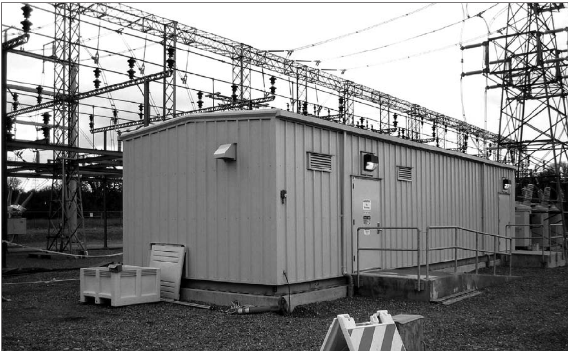
Fig 1. 115 kV single breaker double bus and control building.
