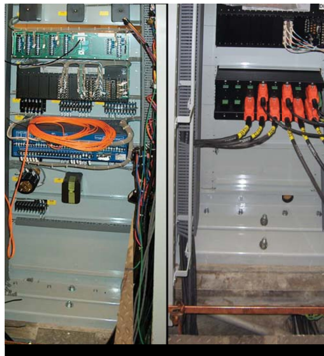
Before (left) and after (right) pictures show a significant reduction in the amount of cabling at relay panels.
