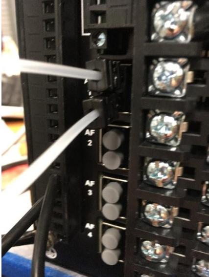
Figure 19 Loop Sensor Incorrect Installation;
