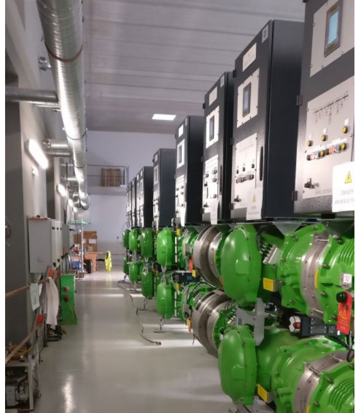
Figure 15: 72.5 kV F35 GIS using g^3 installed in RTE's Grimaud substation in France
