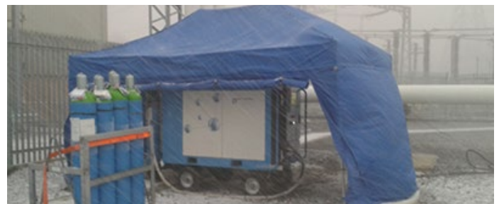
Figure 11: g 3 -filling under harsh weather conditions of the 420 kV GIL for Scottish Power's Kilmarnock substation, UK
