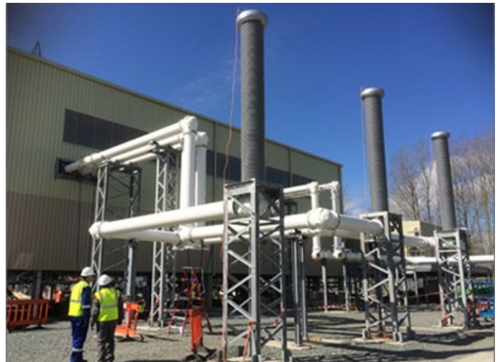
Figure 2: A 420 kV gas-insulated line filled with g^3 at National Grid's new Sellindge substation in the UK
