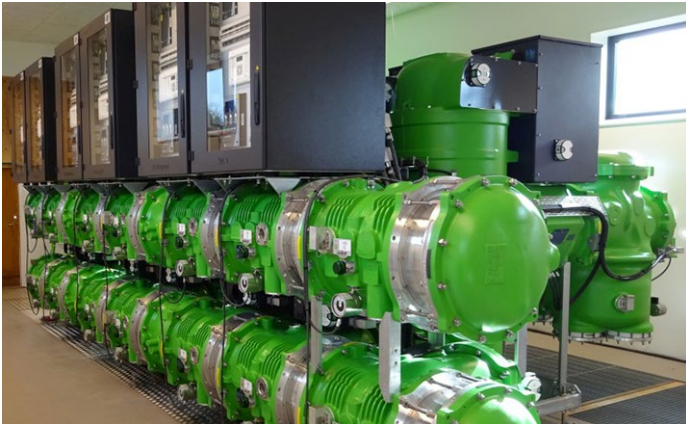
Figure 1: CERIOUS' F35-72.5 kV g^3 gas-insulated substation, including six circuit-breaker bays, is located in Denmark
