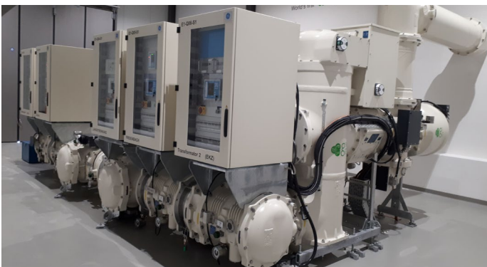
Figure 14: 123 kV GIS with g^3 installed and energized at Axpo's Etzel substation in 2018
