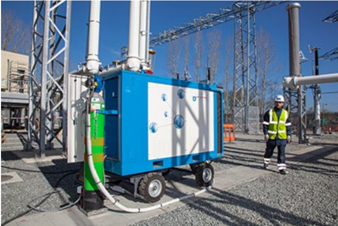
Figure 4: Air Liquide's g 3 -filling cart in service at a National Grid site in the UK
