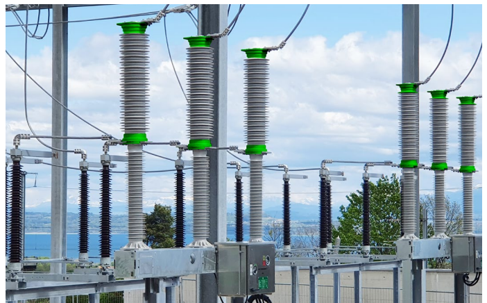
Figure 3: SF_6 -free 145 kV live tank circuit breaker using g^3 switching medium installed at Groupe e's substation in Switzerland.
