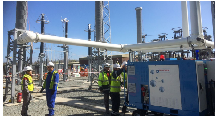
Figure 10: g 3 -filling of the 420 kV GIL at National Grid's Sellindge substation, UK
