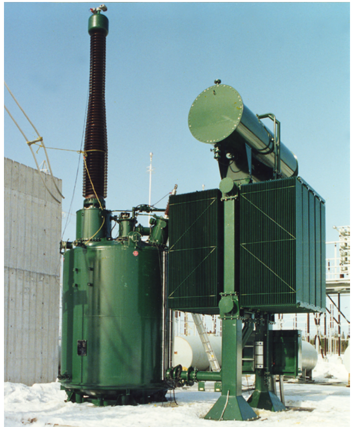
110 Mvar, 765 kV single-phase shunt reactor for Hydro Quebec. Chamouchouane s/s (Canada)
