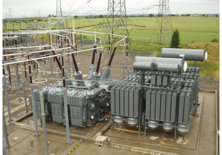
Quadrature Booster 2750 MVA 400/80 kV for National Grid Co. plc. High Marnham (UK)
