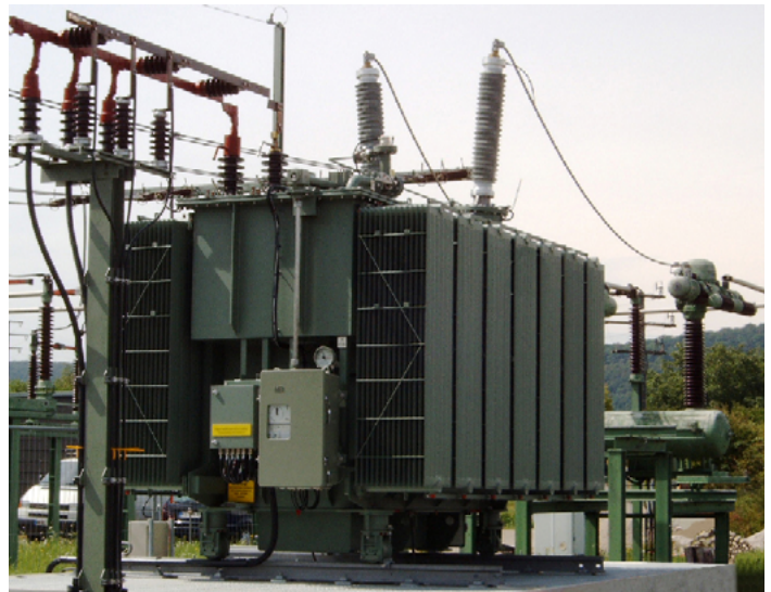
15 MVA 120/17.25 kV hermetic-type trackside transformer for Deutsche Bahn (Germany)
