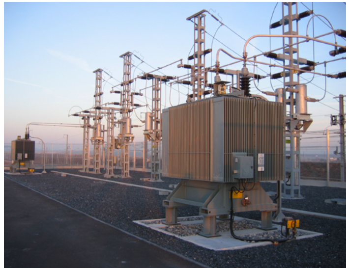
Autotransformers in SNCF railways (France)
