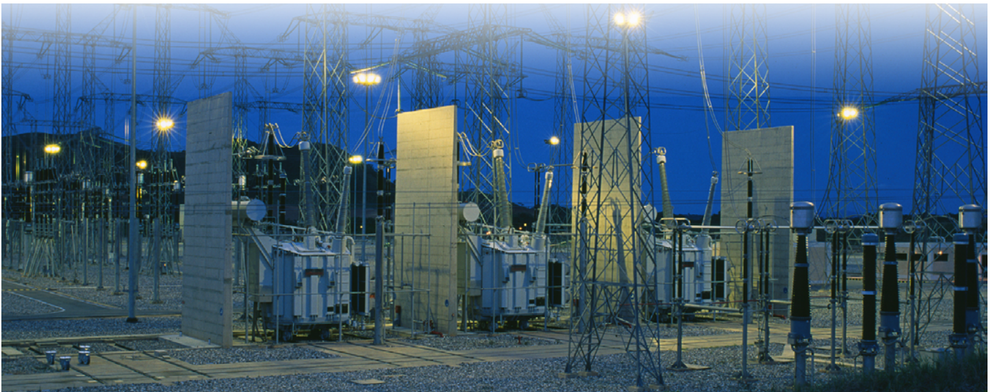
Single-phase autotransformers 500 MVA 765/400/20 kV in operation since the early 80's for EDELCA (Venezuela)
