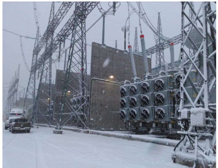
HVDC converter transformer 350 kV DC for Lower Churchill, Canada
