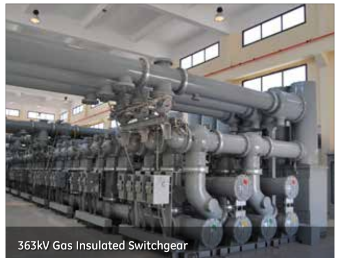
363kV Gas Insulated Switchgear at Golmud Substation
