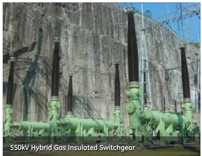
550kV Hybrid Gas Insulated Switchgear
