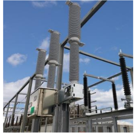
Live Tank CB in Switzerland (Groupe E)
